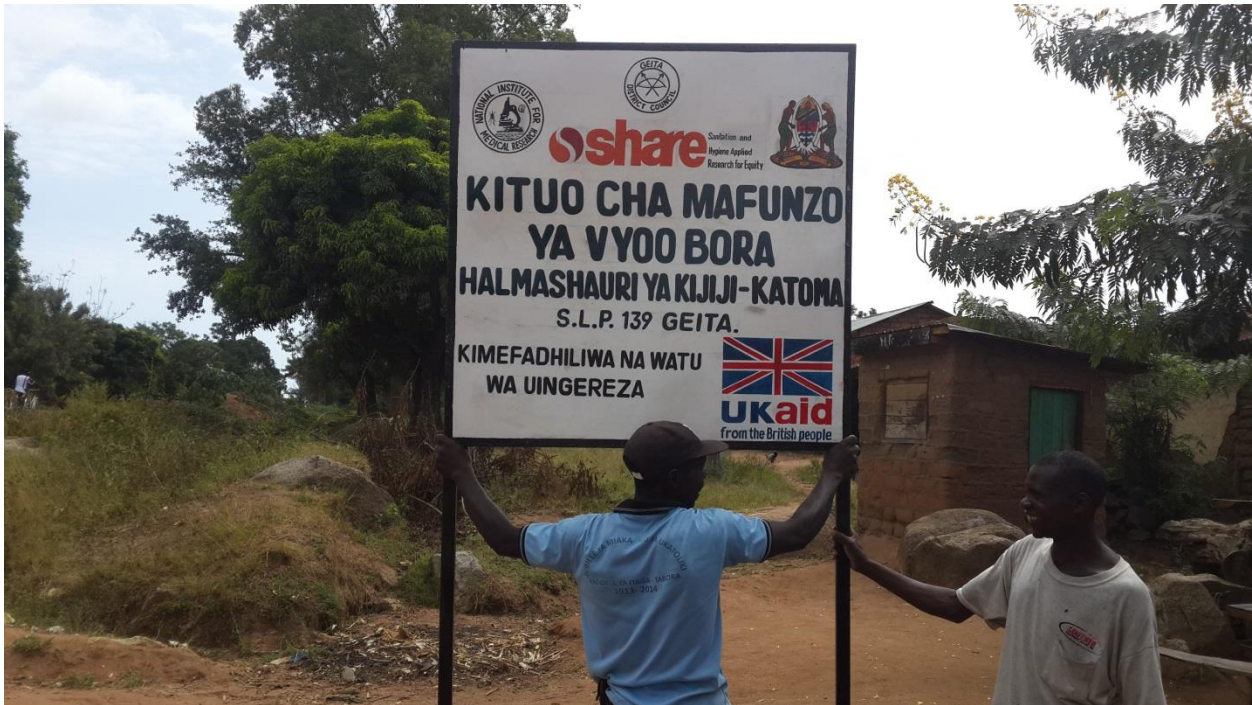
Figure 3: Artisan cementing a sign post that is used to indicate the direction to the sanitation centre at Katoma village in Geita. Photo credit: Yolanda Mbatia
