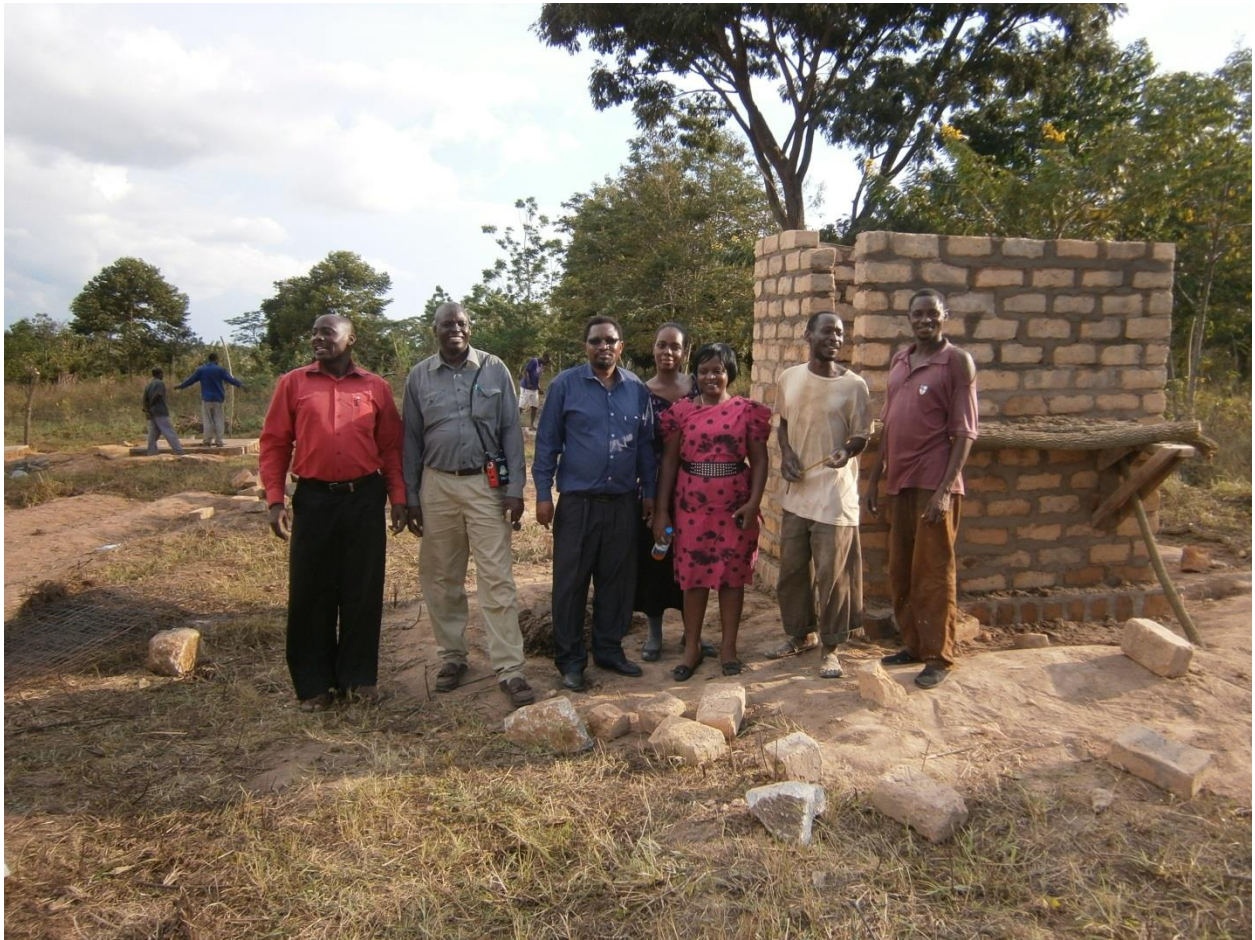
Figure 13: An improved pit latrine model with a squared wall superstructure at the final stages of construction. Photo credit: Jimmy Mtabwa
