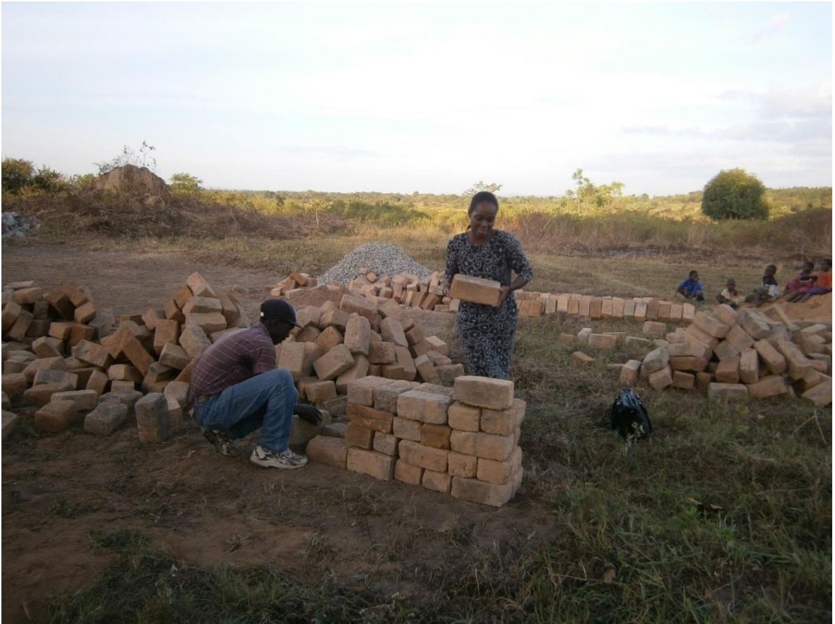
Figure 5: The Principal Investigator of Mtumba Sanitation and Hygiene participatory approach (Mtumba Scale up) – Yolanda Mbatia together with Artisan trainer of trainers (TOT) Stephen John during the preparatory stages of the construction of the sanitation centre at Katoma village. Photo credit: Hamisi Malebo
