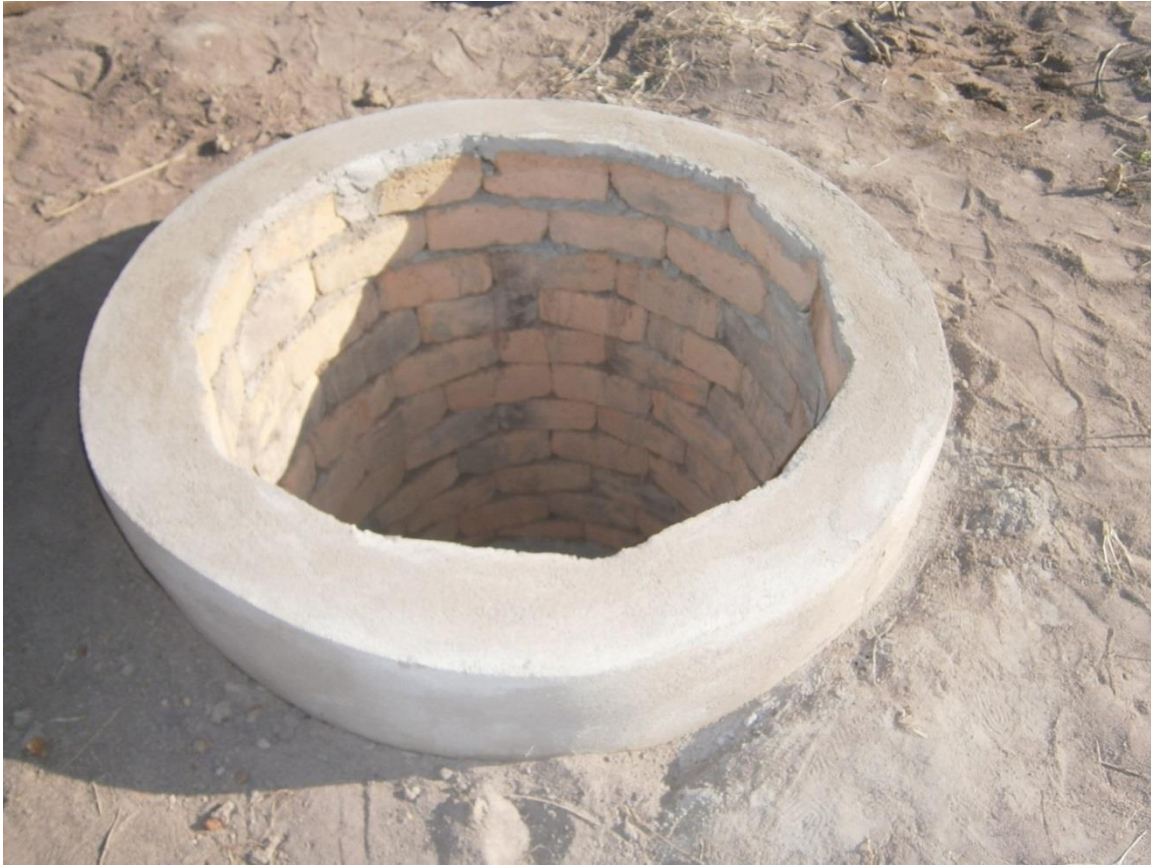
Figure 6: Pit lining model for stable pit walls - stabilized cement blocks placed horizontally. Photo credit: Hamisi Malebo
