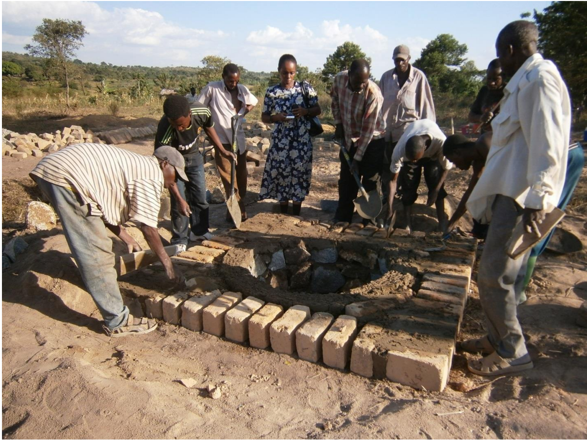
Figure 8: Pit lining model for stable pit walls - stabilized stones. Photo credit: Hamisi Malebo
