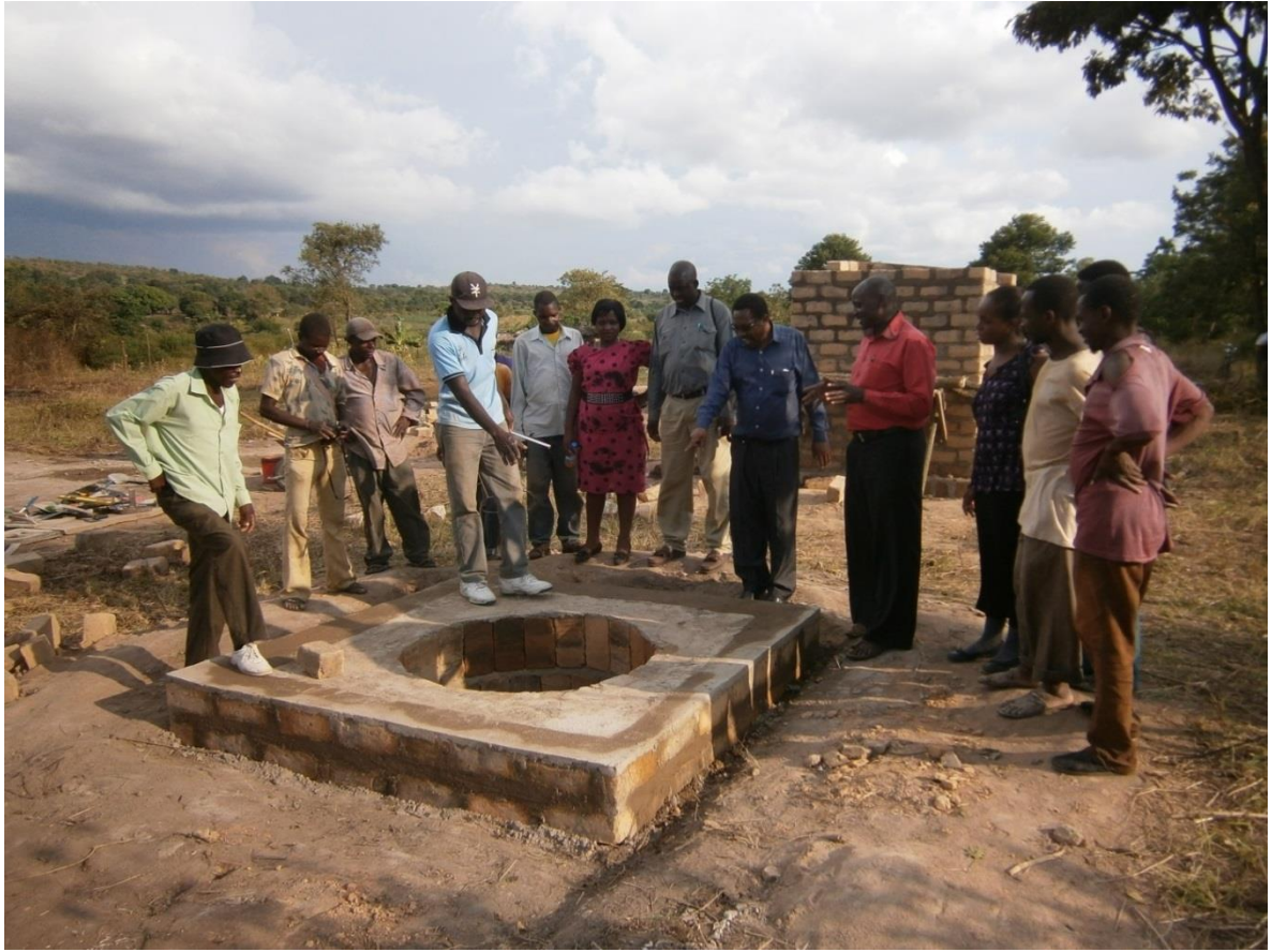
Figure 7: Pit lining model for stable pit walls - stabilized cement blocks placed vertically. Photo credit: Jimmy Mtabwa
