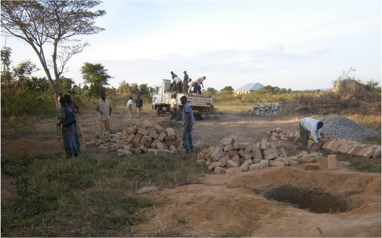
Figure 4: Preparations of a pit model which is an example of a pit to be used in constructing improved latrines. Photo credit: Hamisi Malebo
