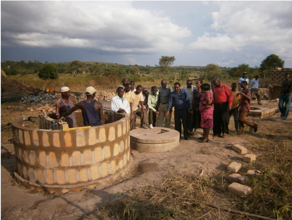
Figure 12: Construction of the superstructure of improved latrine – pour flush off set to pit type. Photo credit: Jimmy Mtabwa
